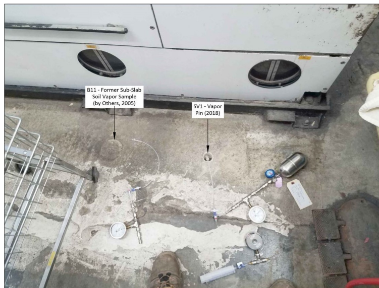
RGI Installed Soil Vapor Pins
